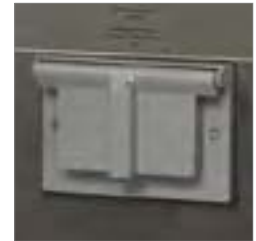
Duplex and/or GFI Outlets
