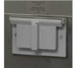
Duplex and/or GFI Outlets
